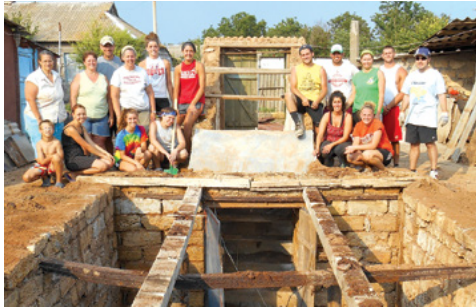
Above and to the right: Widder and volunteers from ComNServ help to restore a building as a part of their Ukraine mission trip.
